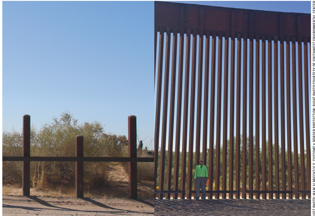
Bollard wall (right) is replacing existing vehicle barriers (left) on the U.S.-Mexico border. (Photos not to scale.)
