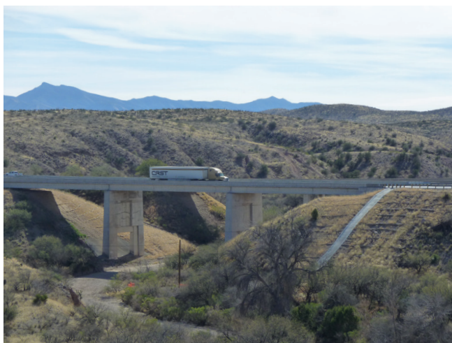
This natural passage beneath I-10 at Davidson Canyon in southern Arizona could allow jaguars to safely cross the busy highway to get to ample suitable habitat on the other side, but the jaguar recovery plan does not address protecting movement corridors across I-10.
