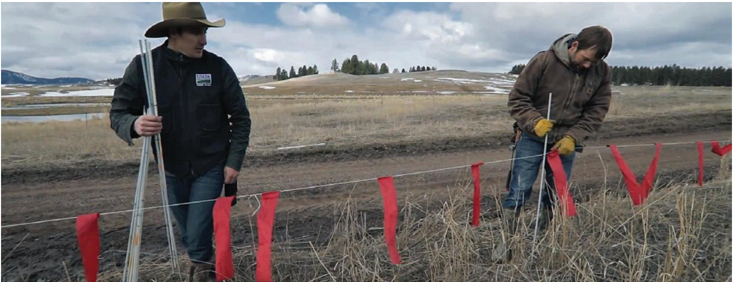
Installing fladry, a rope barrier affixed with red flags that flap in the breeze and scare wolves away.
